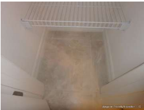
Flooring had paint splatter at the front hallway bathroom closet.
