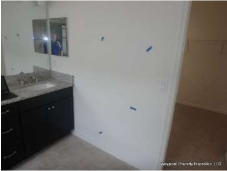
Walls needed touchups at various areas.
