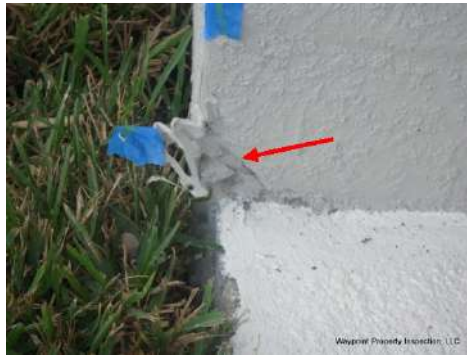
Damage was visible at the rear corner near patio.
