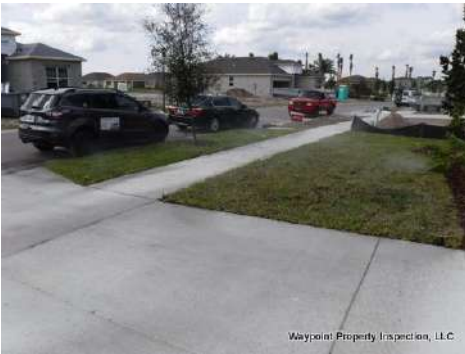
Sprinkler heads should be adjusted for proper coverage.
