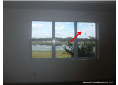
Windows had scuffs at the master bedroom and master bathroom.
