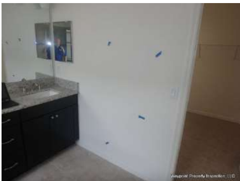
Walls needed touchups at various areas.
