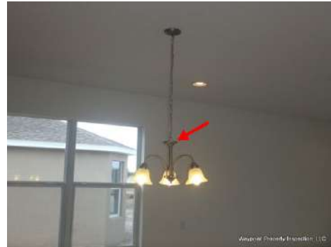
Light fixture was not level.
