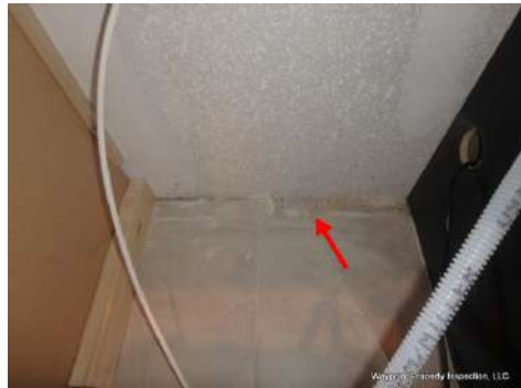
Tile was not installed behind the dishwasher.
