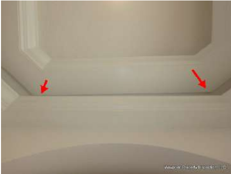
Entry rotunda had poor finish and crown molding/trim was uneven.
