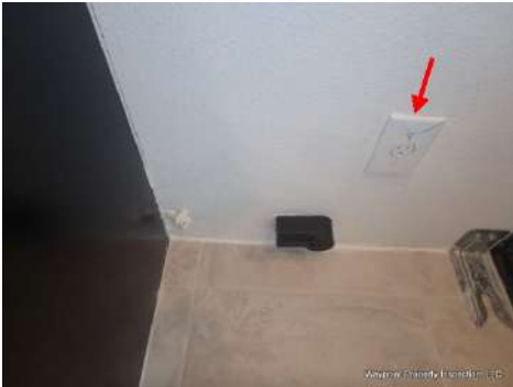
Cover plates were damaged at kitchen oven/stovetop.
