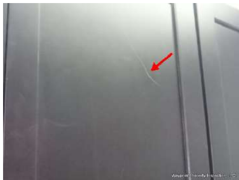
Cabinet doors were scuffed/scratched.
