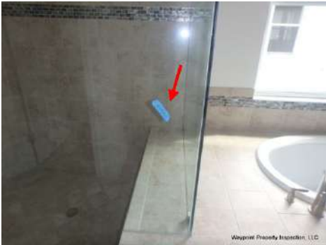
Shower enclosure glass appeared scratched at master bathroom.
