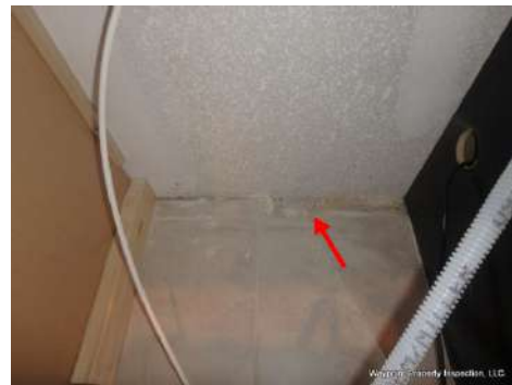
Tile was not installed behind the dishwasher.
