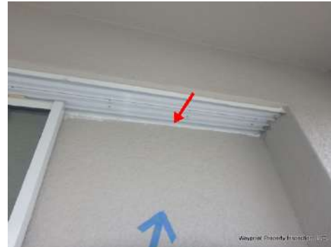
Sliding door jamb needed sealant and paint.
