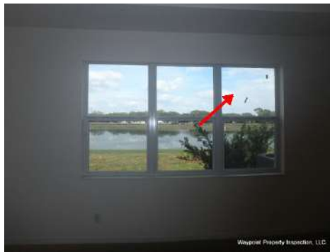
Windows had scuffs at the master bedroom and master bathroom.
