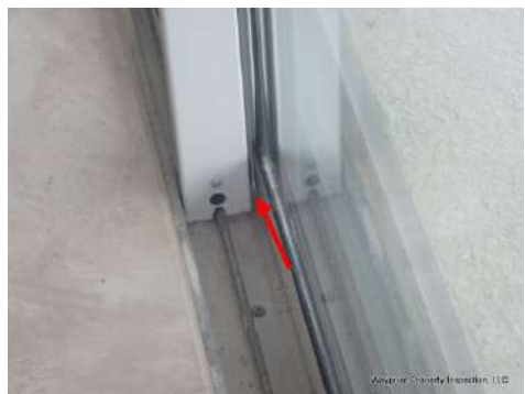
Sliding door had visible gaps at the base.
