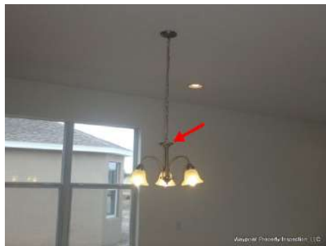
Light fixture was not level.
