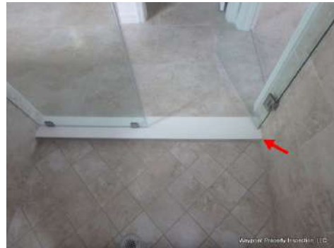
Grout was needed at shower walls at master bathroom.
