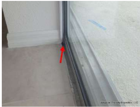
Sliding door had visible gaps at the base.
