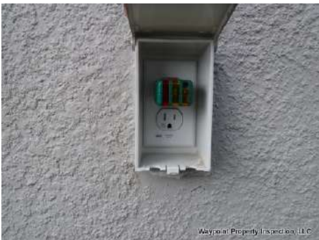
GFCI outlets did not operate when tested at exterior right side and rear outlets.
