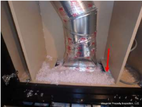
Gaps around kitchen ventilation should be sealed. Visible insulation was fell through.
