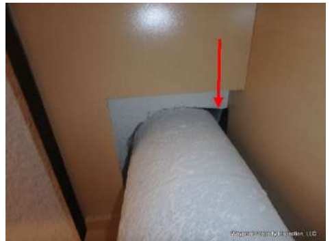
Gaps around kitchen ventilation should be sealed. Visible insulation was fell through.
