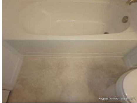
Bathtub trim was loose at hallway bathroom (rear) and hallway bathroom (front).
