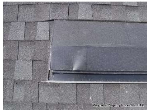
Roof vent had minor damage.
