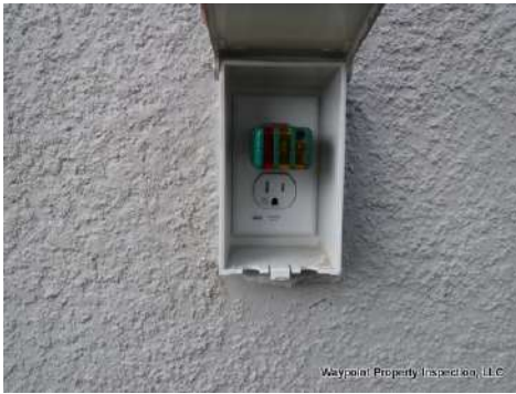
GFCI outlets did not operate when tested at exterior right side and rear outlets.
