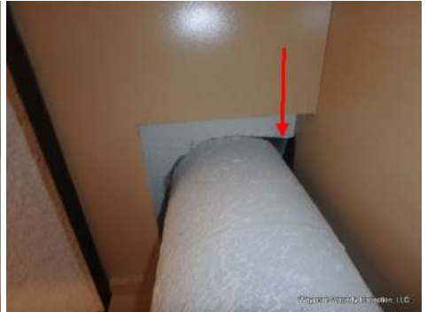
Gaps around kitchen ventilation should be sealed. Visible insulation was fell through.
