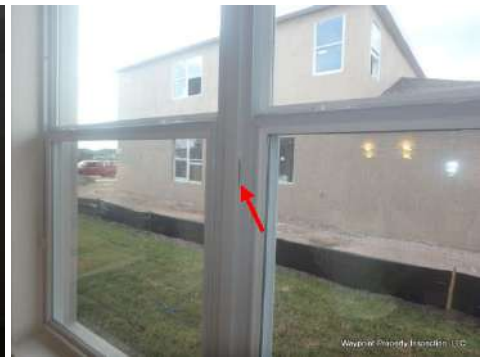
Window was damaged at the kitchen dining area.
