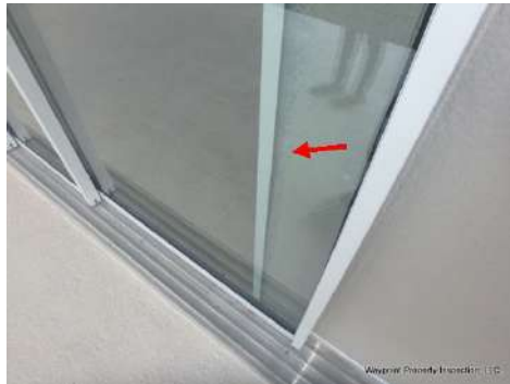
Sliding door jamb needed sealant and paint.
