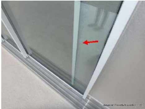
Sliding door jamb needed sealant and paint.
