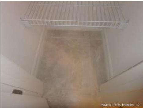
Flooring had paint splatter at the front hallway bathroom closet.
