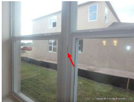
Window was damaged at the kitchen dining area.
