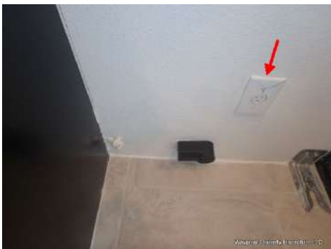
Cover plates were damaged at kitchen oven/stovetop.
