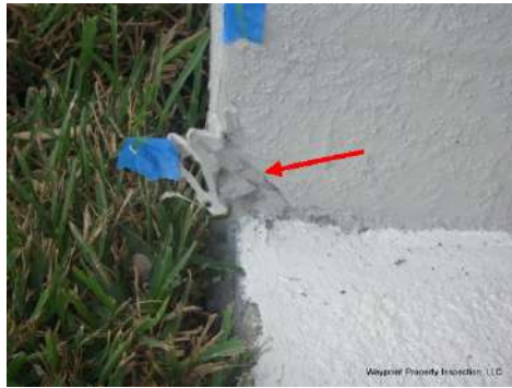
Damage was visible at the rear corner near patio.
