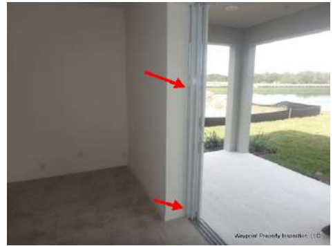
Sliding door was not level when doors were fully opened.
