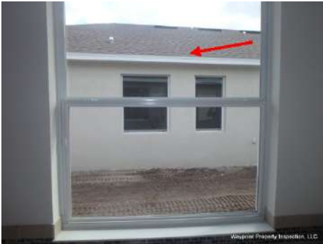
Windows had scuffs at the master bedroom and master bathroom.
