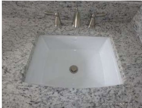
Drain stopper was not functioning at master bathroom right side.
