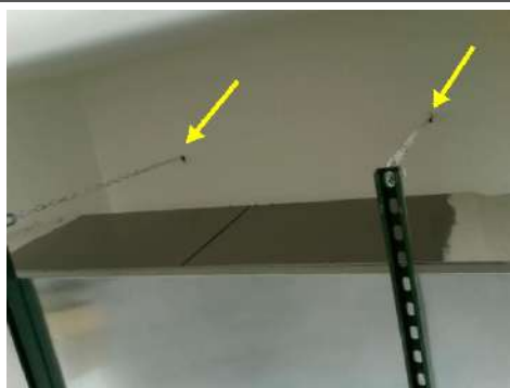
Holes/gaps should be sealed with fire rated sealant.
