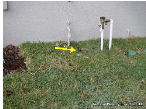
Sprinkler heads should be adjusted for proper coverage.
