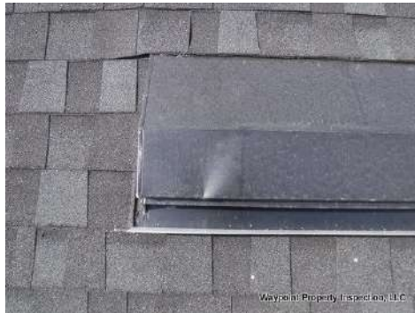
Roof vent had minor damage.
