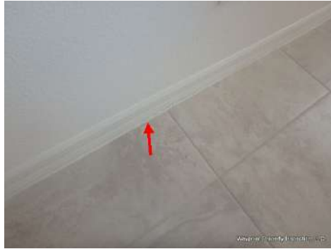
Baseboards should be caulked at the dining room.
