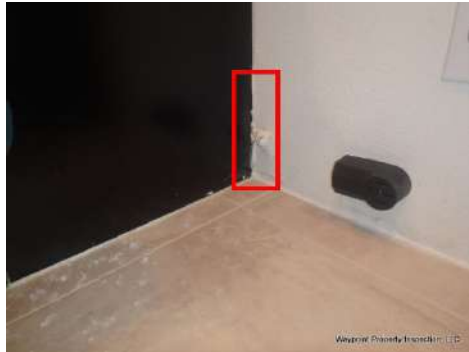
Wall at kitchen range gas piping should be sealed.
