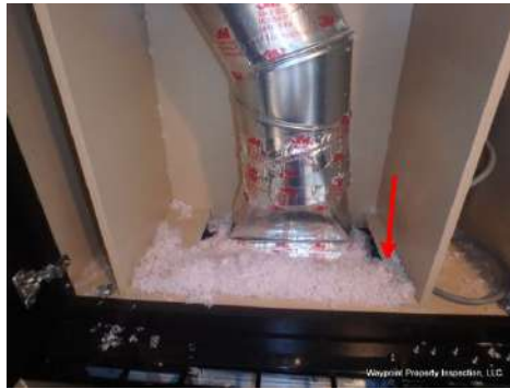
Gaps around kitchen ventilation should be sealed. Visible insulation was fell through.
