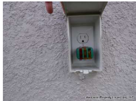
GFCI outlets did not operate when tested at exterior right side and rear outlets.
