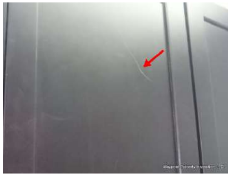
Cabinet doors were scuffed/scratched.
