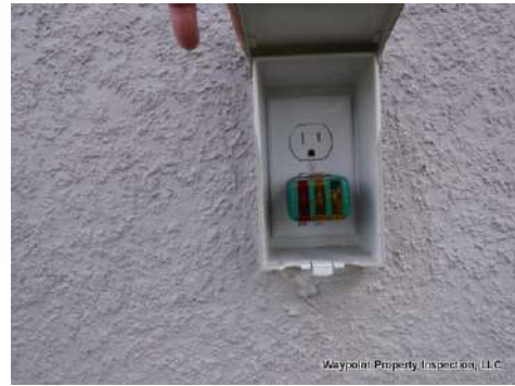
GFCI outlets did not operate when tested at exterior right side and rear outlets.
