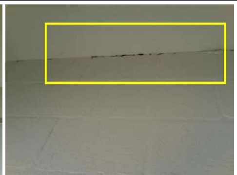
Holes/gaps should be sealed with fire rated sealant.
