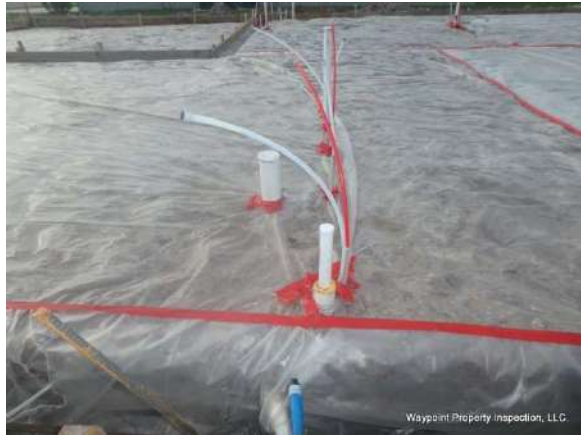
Main line / Plumbing penetrations
