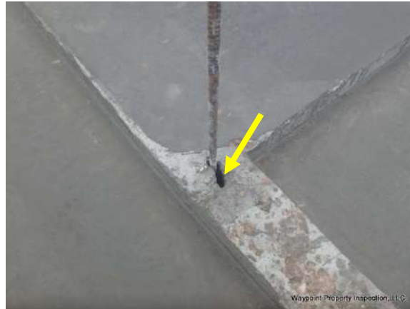
Rebar penetration at the porch area had visible gap
